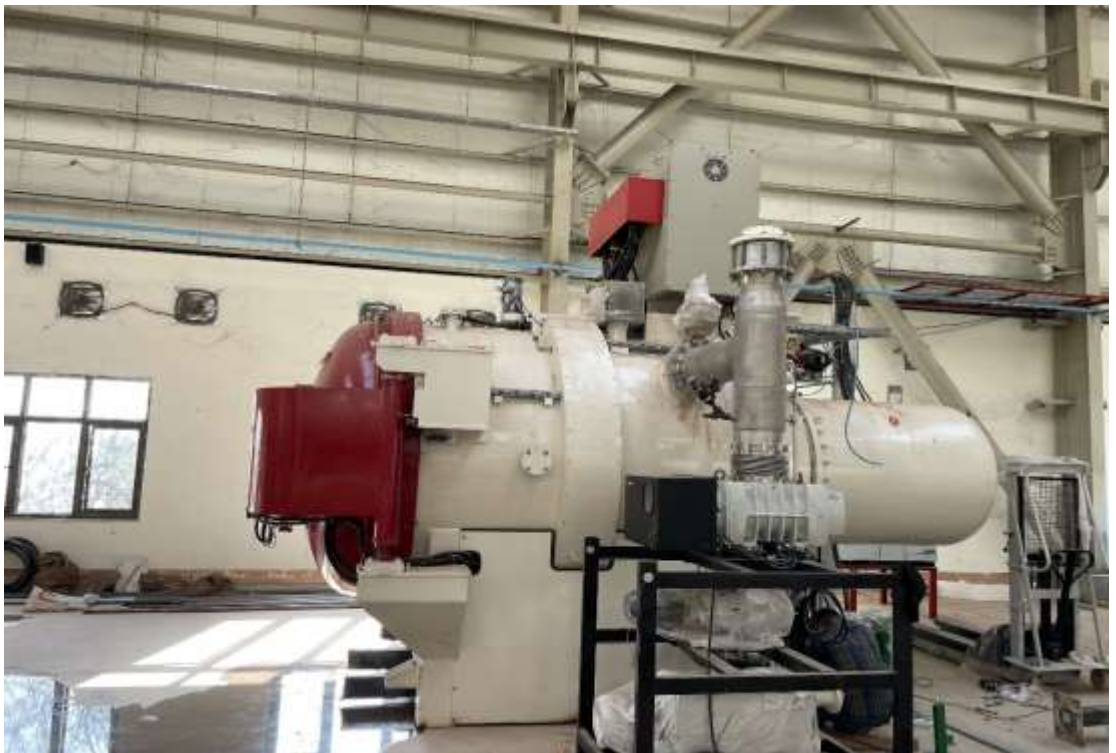
Vacuum Heat Treatment Furnace
